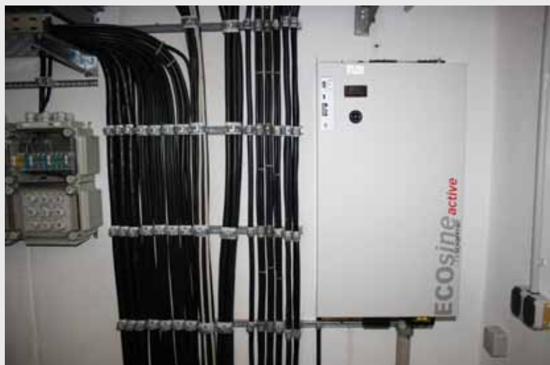
Advanced active harmonic filter installed in transmission station
