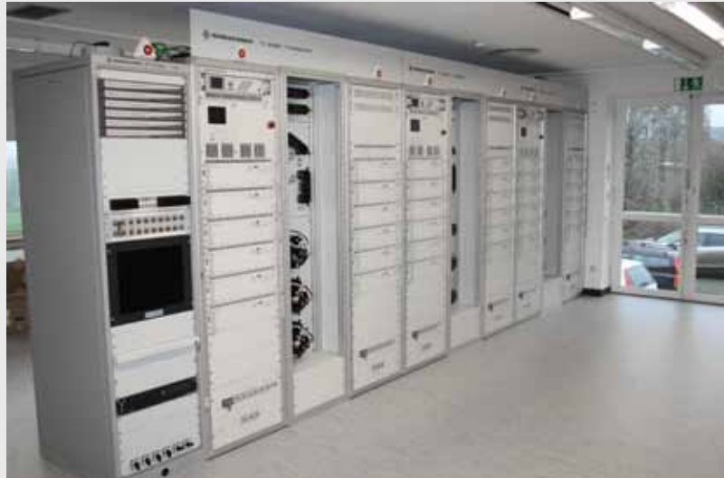
Part of DVB-T transmission station
